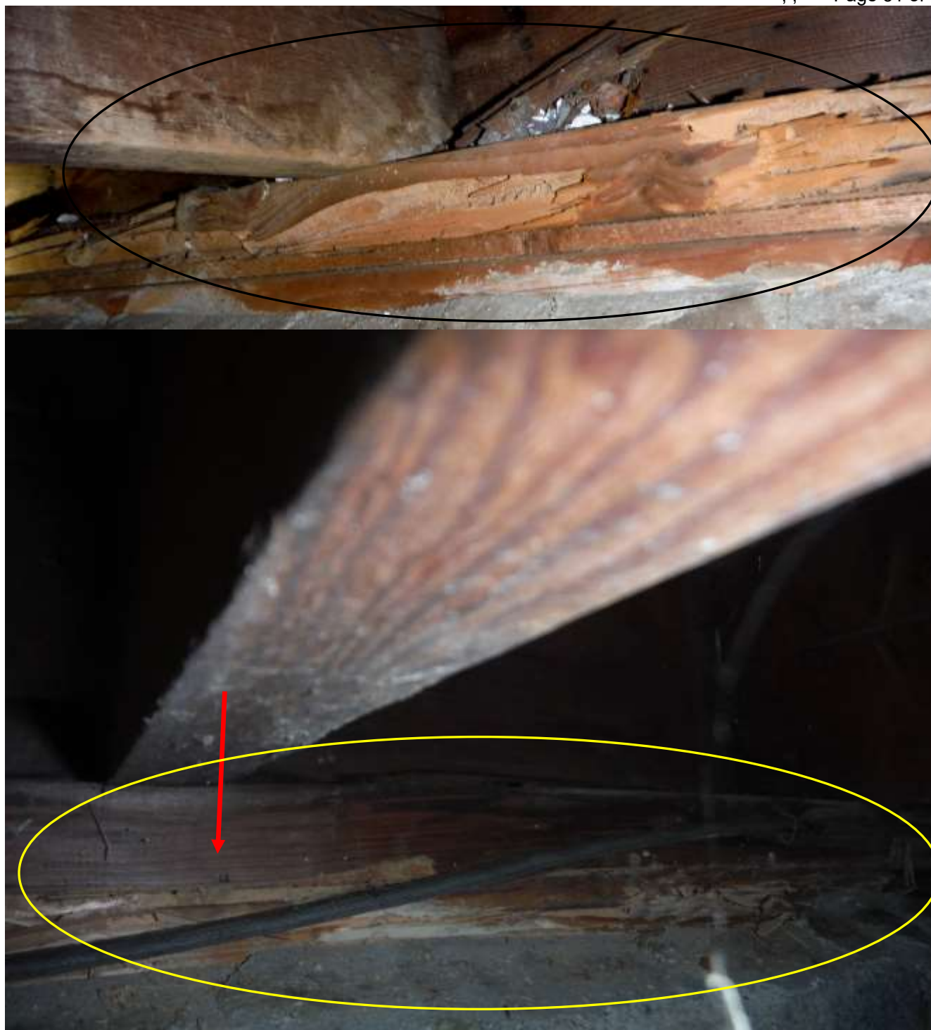
Figure 3 Joists compressing termite damaged sills; structural/material defects.
