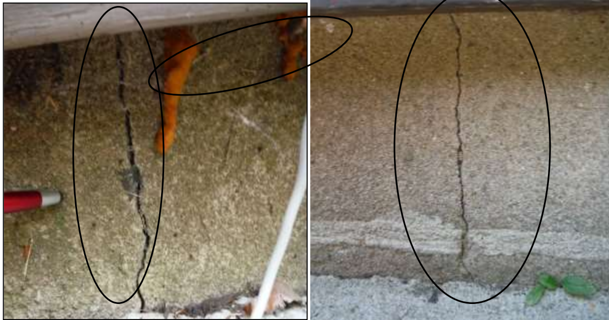
Figure 1 Examples of foundation cracks; have evaluated by a structural mason and/or engineer (PE).
