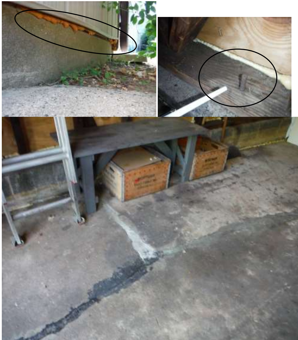
Figure 2 Damage to floor & foundation visible in garage; have a structural mason or qualified foundation repair contractor and/or structural engineer evaluate the homes structure ( cracks & termite damage).
